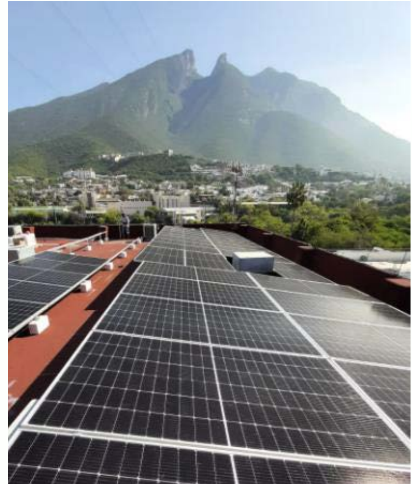
Solar panels at the Monterrey branch in Mexico reduce energy usage and cost
